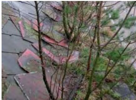
Weathering issues affecting the building surfaces, such as humidity and plants.
