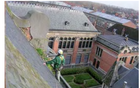
Assessing the roof of a heritage place using industrial rope access techniques
