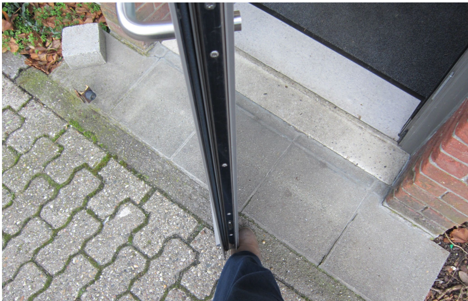
Figure 8. Heavy emergency exit door with a paving stone (left) to keep it open at night.
