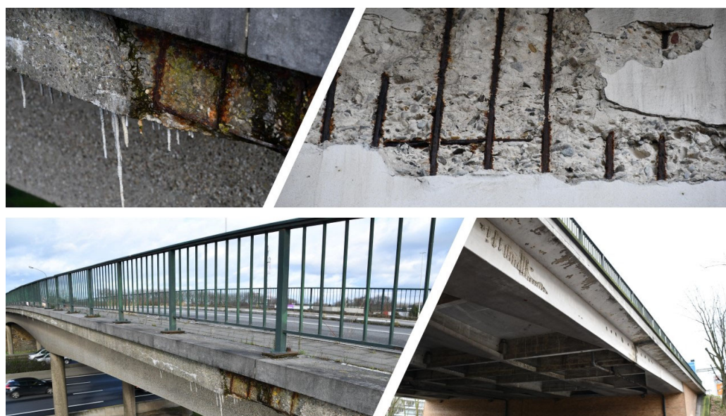
Figure 1. Examples of concrete spalling due to reinforcement corrosion.
