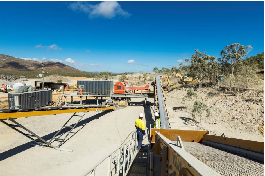
Figure 2: Pilot X-ray sorter installed in Mt Carbine – courtesy of EQ Resources
