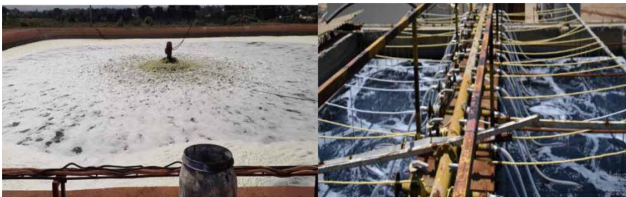
Figure 3 | Aerated biological units.
