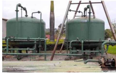
Figure 4 | Activated carbon filters.
