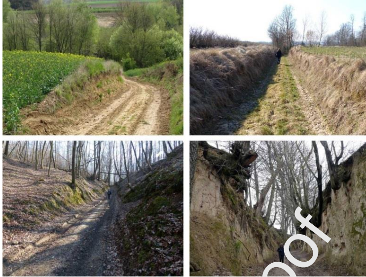
Figure 7. Active sunken lanes. Illustration of successive downcutting stages of unpaved roads by traffic and water erosion in the western part of Nieleczów Plateau (E Poland) (Photo: W. Zgłobicki).
