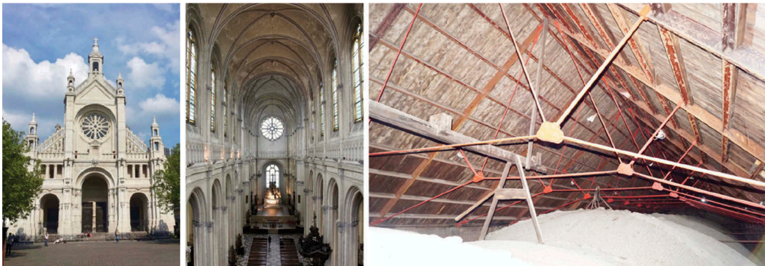
Figure 9. St. Catherine's church (1851–66) in Brussels. Exterior, interior and trusses (1865–66) (pictures R. Wibaut).
