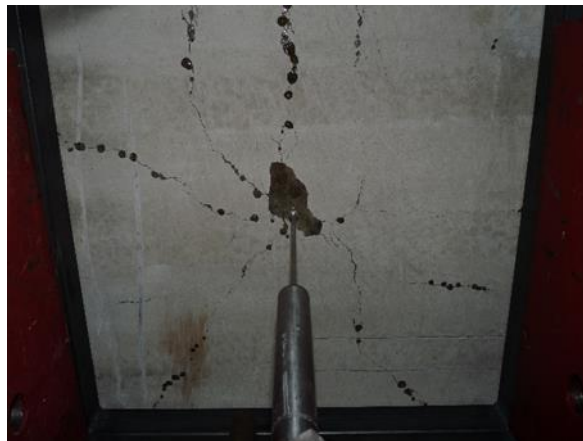
Figure 15. 2D vascular network releasing sodium silicate in a 600mm square concrete slab.
