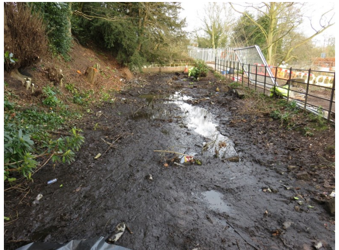
Figure 8b. de-watered, silted section of Rising Brook upstream of weir, lacking white-clawed crayfish
