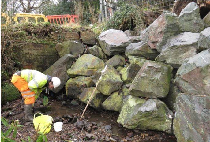
Figure 8d. shallow pools where crayfish collected at the foot of boulders supporting the dilapidated bridge
