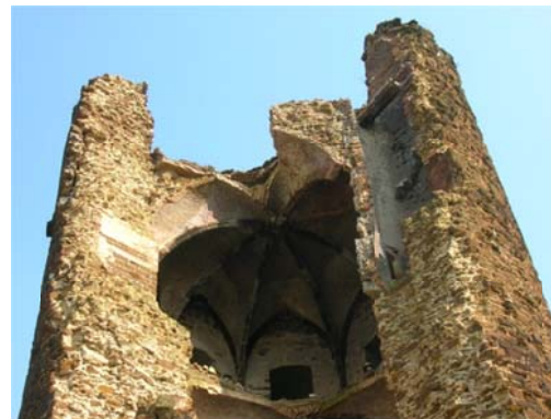
Fig. 2. Maagden tower at Zichem (Belgium), after its partial collapse in 2006.
