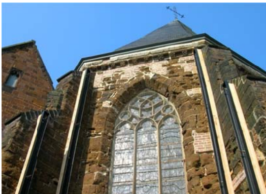
Fig. 1. Severely weathered Diestian ferruginous sandstone with stone replacements made in clay bricks (choir section of the St. Eustachius church at Zichem, Belgium).
