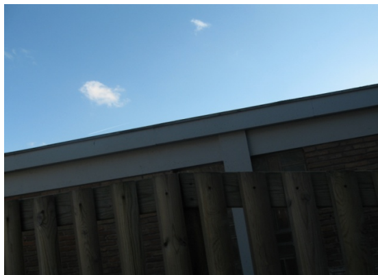
Figure 10. Picture of the sloping surface in the playground
