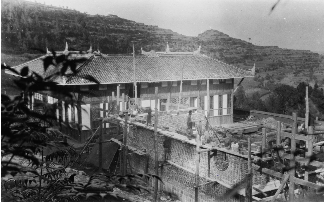
Fig. 2. Priory of Xishan under construction, ca 1929 (Archives of the Abbey of Maredsous).
