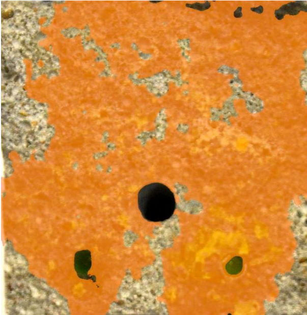
Fig. 17. Crack surface (40 x 40 mm 2 ) of one of the specimens with the best PU surface coverage but still a significant flow due to an unconnected crack filling below the cast-in hole (through which water was induced during the permeability test). The crack mouth through which water leaked out of the specimen is oriented to the bottom, like in the water flow test.
