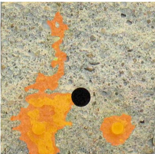
Fig. 18. Crack surface (40 x 40 mm 2 ) of specimen with limited PU surface coverage.
