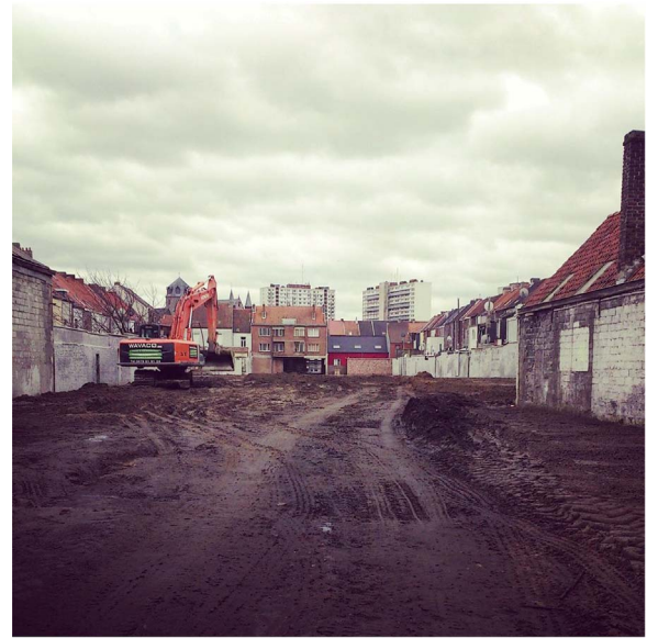
Fig. 2. The Boerenhof in February 2014 after the mishmash of garage boxes and other structures were cleared.
