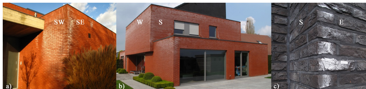
Figure 1 Efflorescence develops preferentially on a), b) facades and c) edges which are exposed to an intensified action of rain and wind. The capital letters indicate orientation of the facades: S – south, W – west, E – east.
